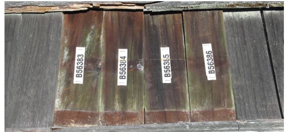
○ Flat panels Abodo Vulcan Radiata 230°C after 11 years exposure, Rotorua.
